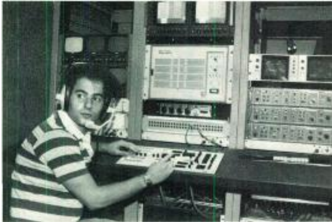
Do-it-yourselfer Victor Cognato, video engineer for Valley Cable TV, put $80,000 worth of equipment in a step van "home-built" that he configured for Valley's needs.
